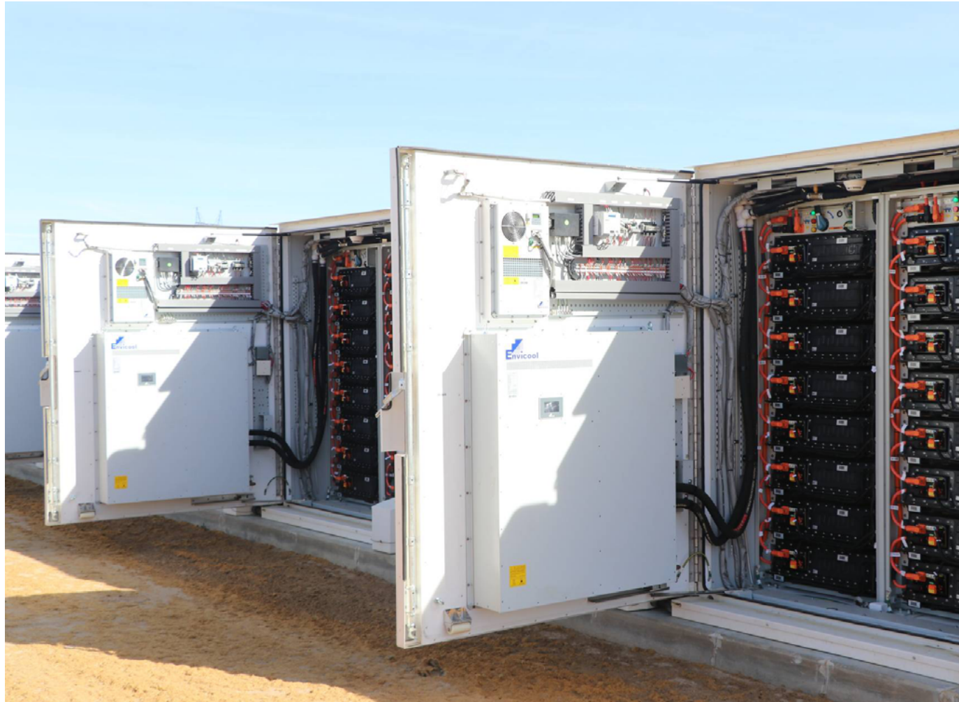
The 100 MW / 400 MWh Luna battery storage facility came online in August 2022 and provides enough energy to power roughly 75,000 Southern California homes for four hours every day.
